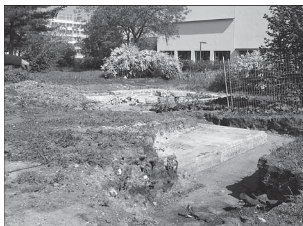
Figure 9: Excavation works in Dresden revealed some interesting aspects of the former park design (source: Dresden, 2006).
